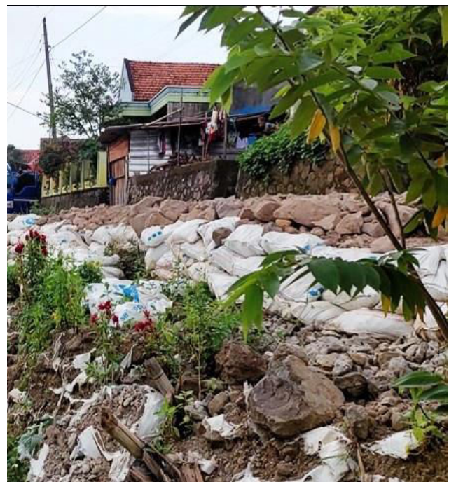
Figure-1. Community and local government efforts to deal with road subsidence as putting stakes and sand in sacks.
