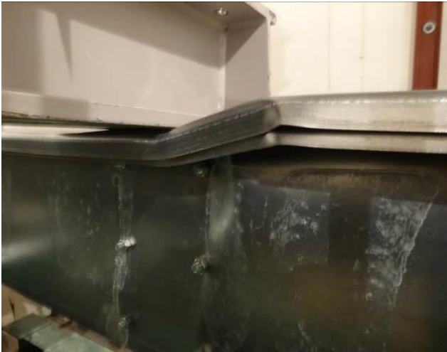
Figure-11. Detail of Z-purlins damage.
